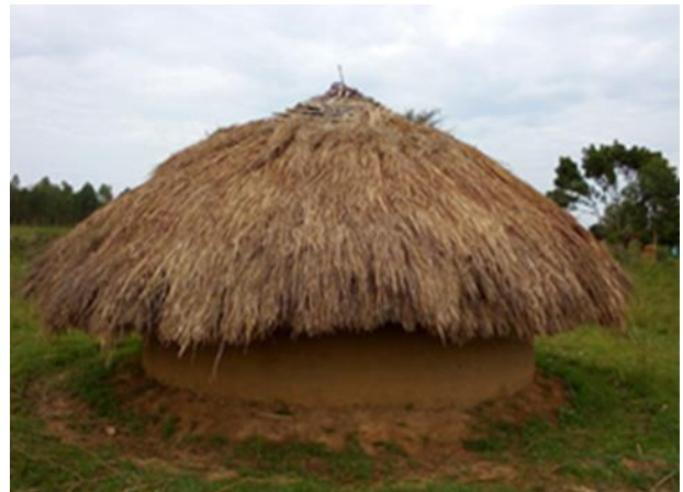
Fig. 2. Most of the children who were injured were attempting to take shelter from the drizzle by sitting on a small veranda or bench seen at the base of this unfinished hut. The top center point of the roof was not yet thatched so that rain and sunlight could penetrate to the inside.
