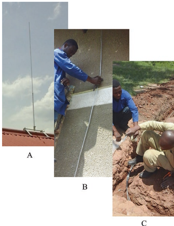
Fig. 17.1 Installation of (a) air terminal, (b) down conductor, and (c) ground terminal at school in Uganda. (Courtesy of ACLENet)
