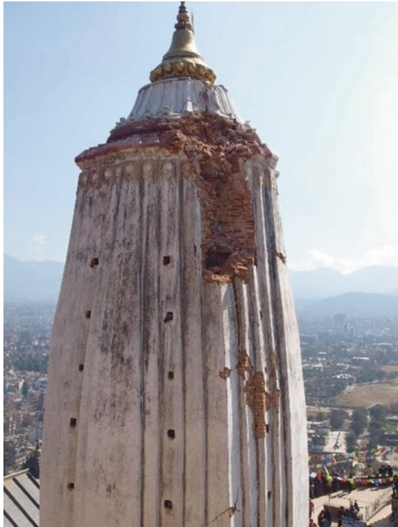
Fig. 5.3 Lightning damage to a historic temple in Nepal. (Courtesy Shri Ram Sharma)
